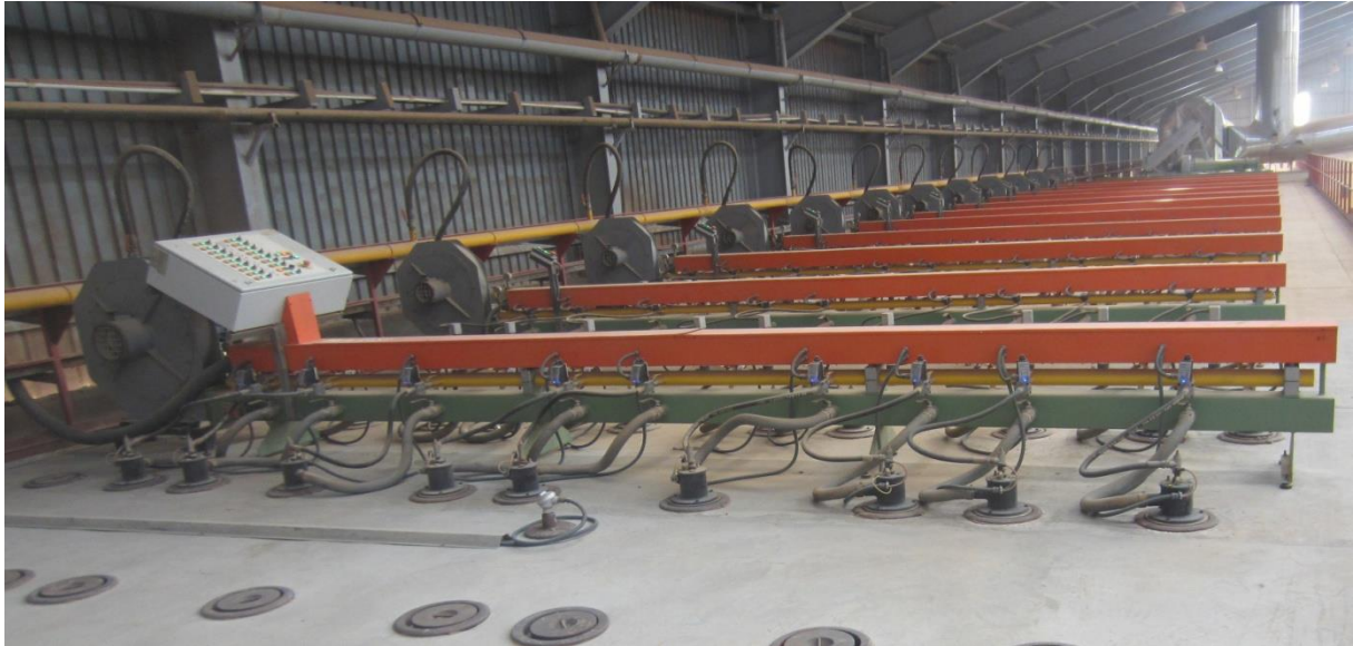
Fig.III.4: Continuous furnace of the factory.
