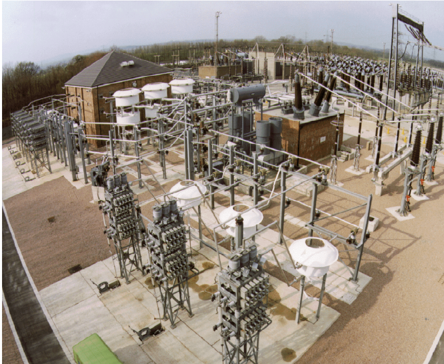
Figure (2.3): SVC 400kV -75/+150 MVar
