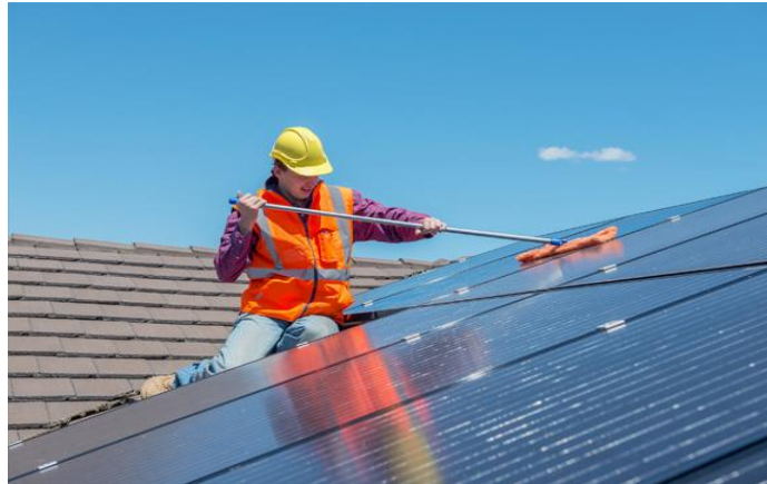
Figure II. 27: Nettoyage des panneaux
