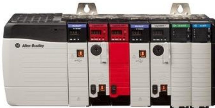
Figure III.1: Programmable logic controller (Allen Bradley)
