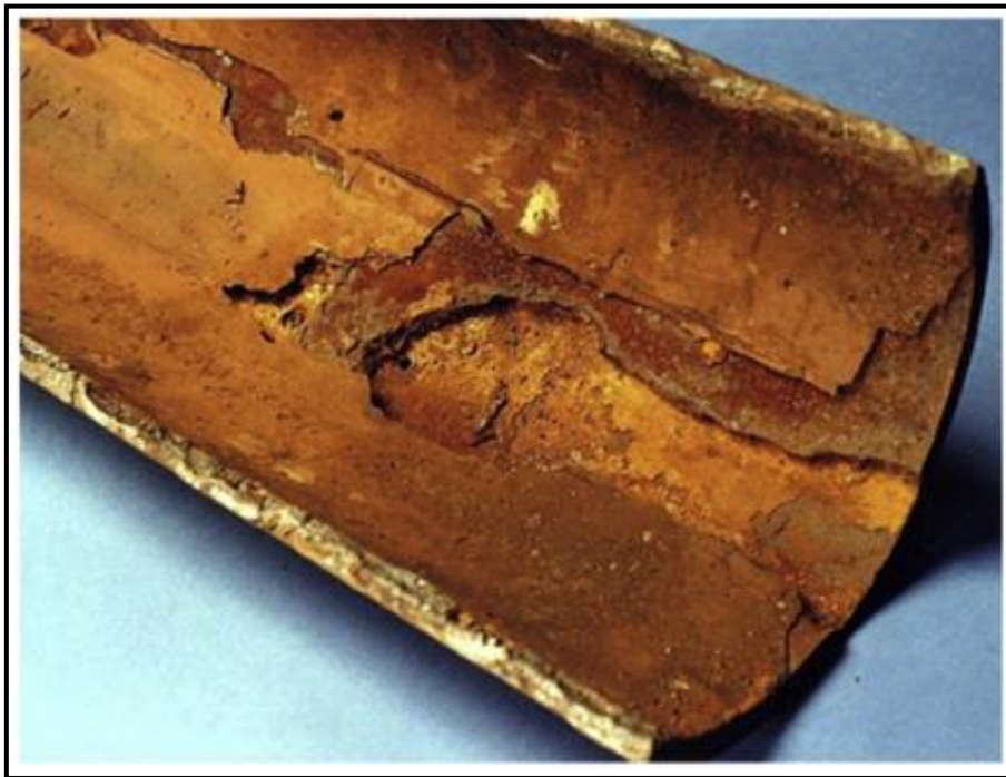
Figure I. 4: Sweet corrosion (CO 2 corrosion) [27].
