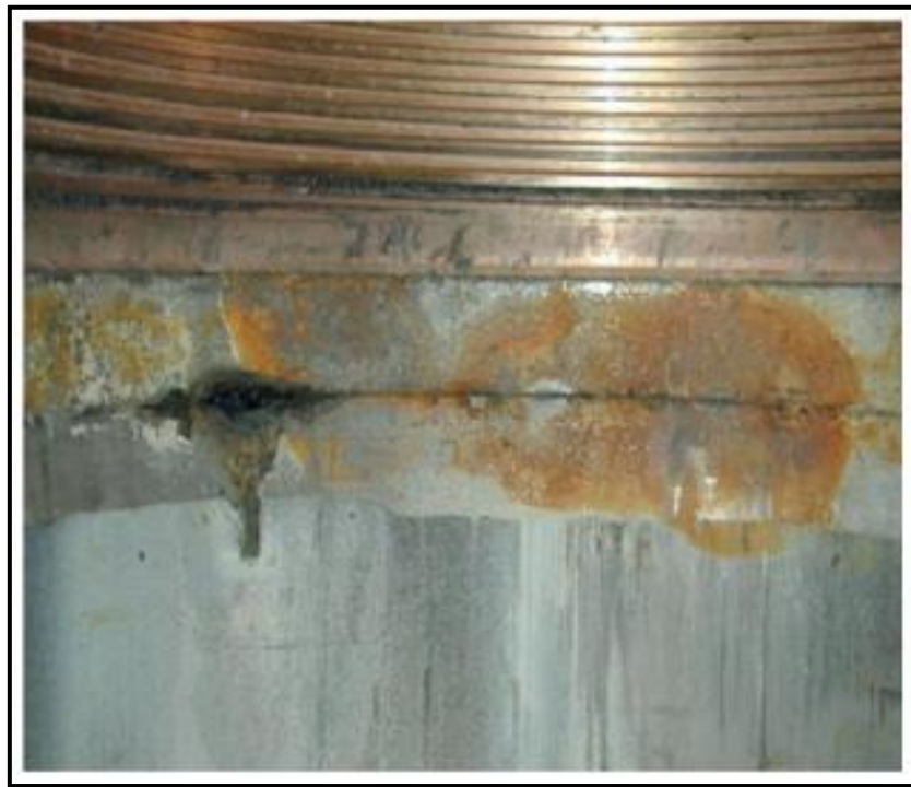
Figure I. 6: Oil and gas pipeline under crevice corrosion [28].
