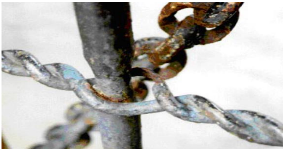
Fig. I.1. A picture that shows corrosion [4].
