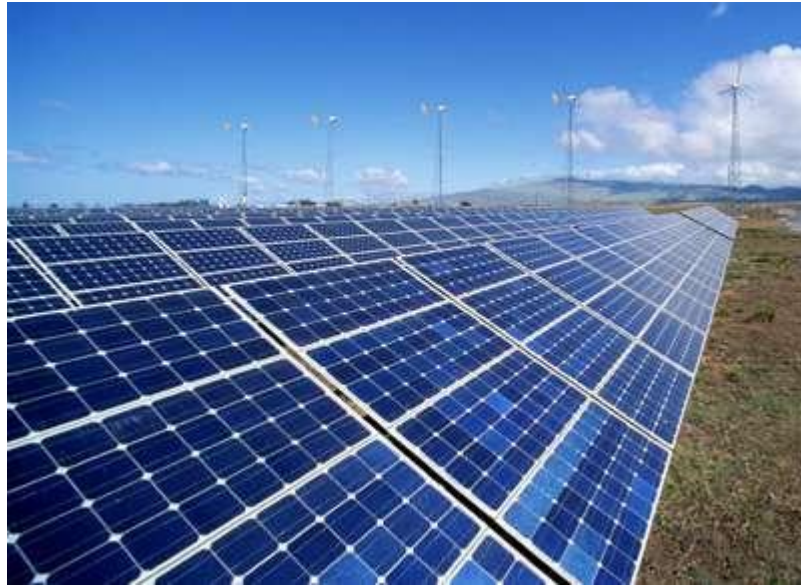
Figure I-2 un champ photovoltaïque
