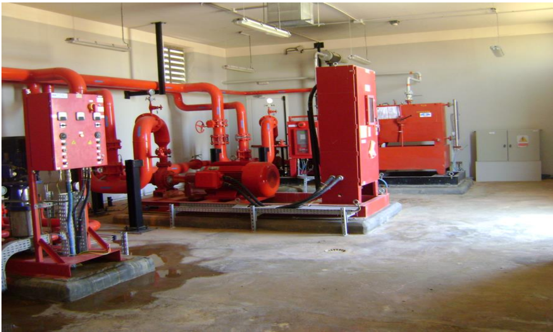
Figure III14 : local pomperie incendie
