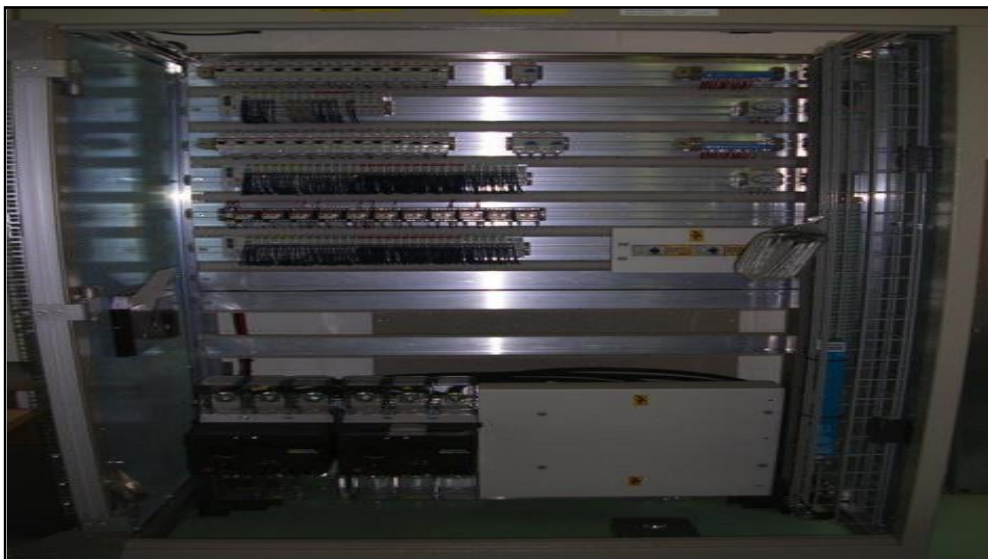
Figure IV.7: L'armoire distribution 230 V
