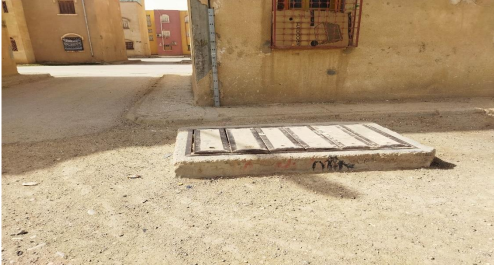
Figure 3.8: Manhole to pass optical fiber.
