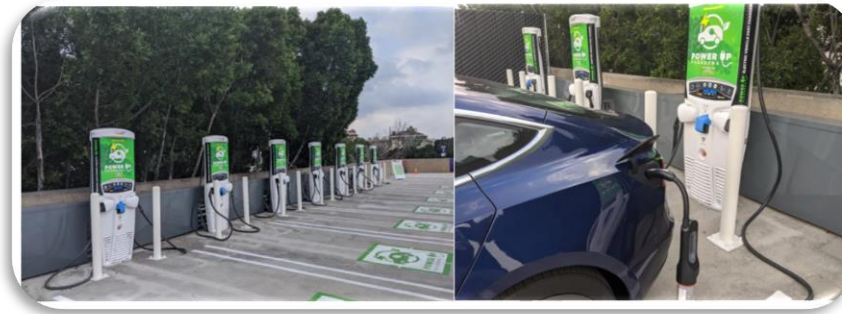
Figure 4 charging stations https://cleantechnica.com/2020/02/17/largest-ev-fast-charging-station-in-the-us-opens-in-pasadena-california/ .2023
