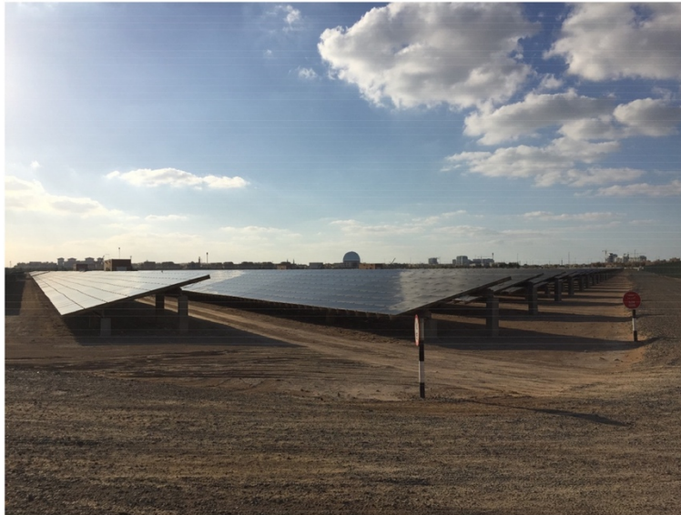
Figure 17: A 10 Megawatt(MW) solar photovoltaic power plant at Masdar City
