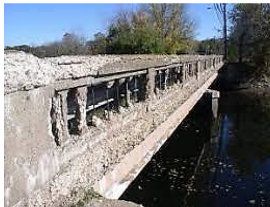
Figure II. 3 Photo of the concrete bridge subjected to spalling [57].
