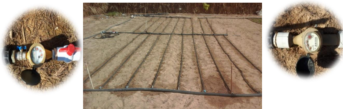
Photo 4: Irrigation network (Original photo 2023)
