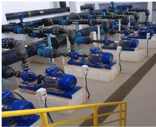
Figure III.30. Treated water pumps
