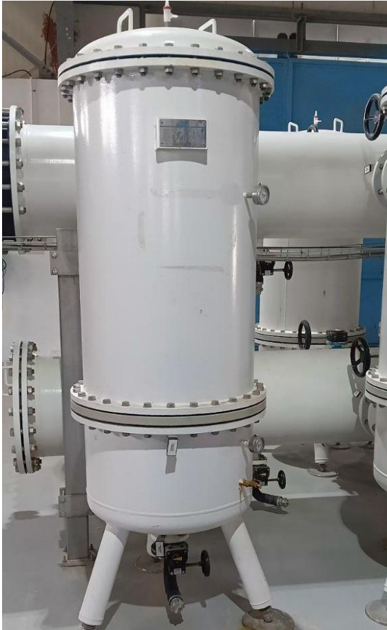
Figure III.27. A cartridge filter unit
