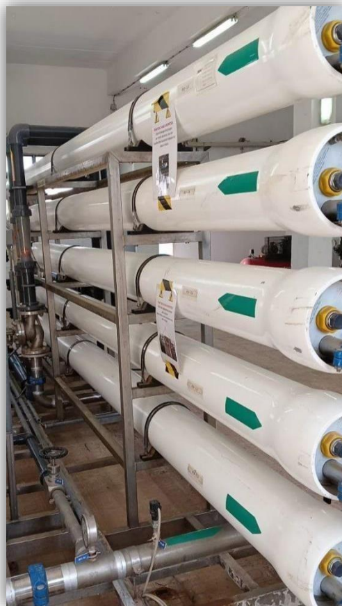
Figure III.6. Reverse osmosis modules at the station
