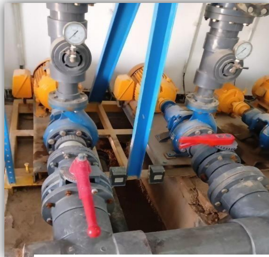
Figure III.4. The sand filter feed pumps
