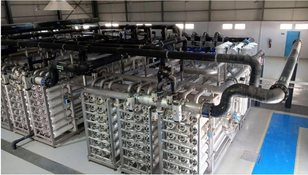
Figure III.29. The station's Reverse Osmosis plant
