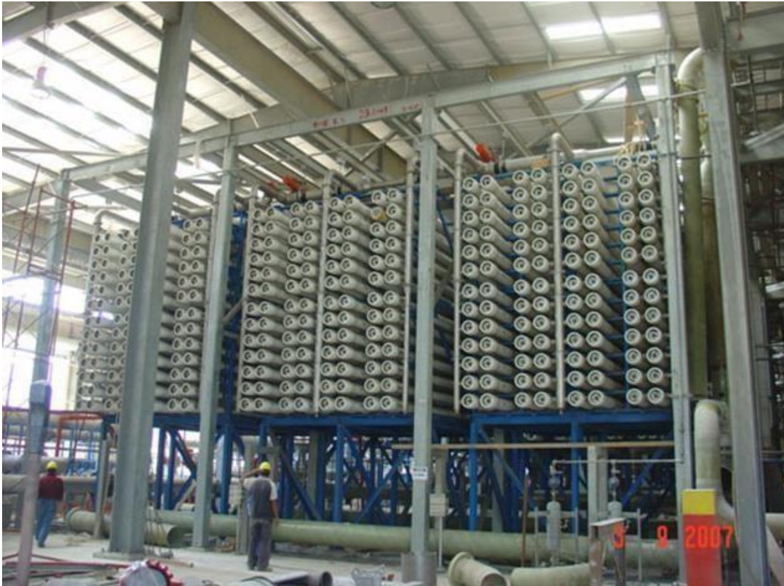
Figure II.1. El-Hamma station's RO units (spa, 2024)
