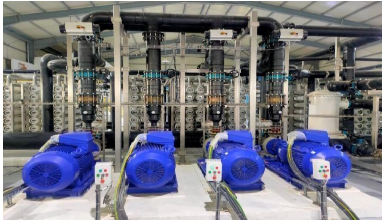
Figure III.28. high-pressure feed pumps.
