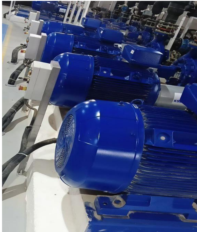
Figure III.24. Low pressure supply pumps
