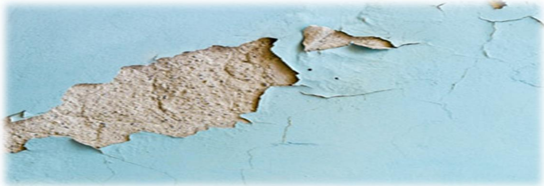
FIGURE 5 ALTERATION PEINTURE DE FACADE
