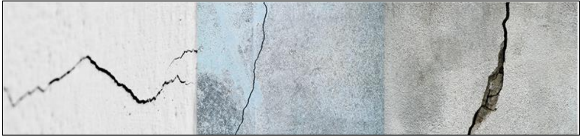
FIGURE 2 :FORMES DE FISSURES
