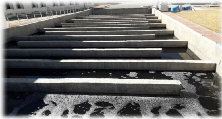
Photo III.13: Bassin de chloration.
