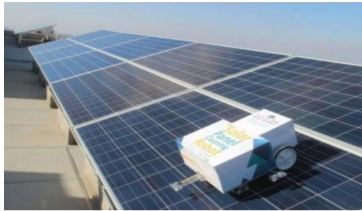
FIGURE III.4 – Nettoyage intelligent des panneaux PVs
