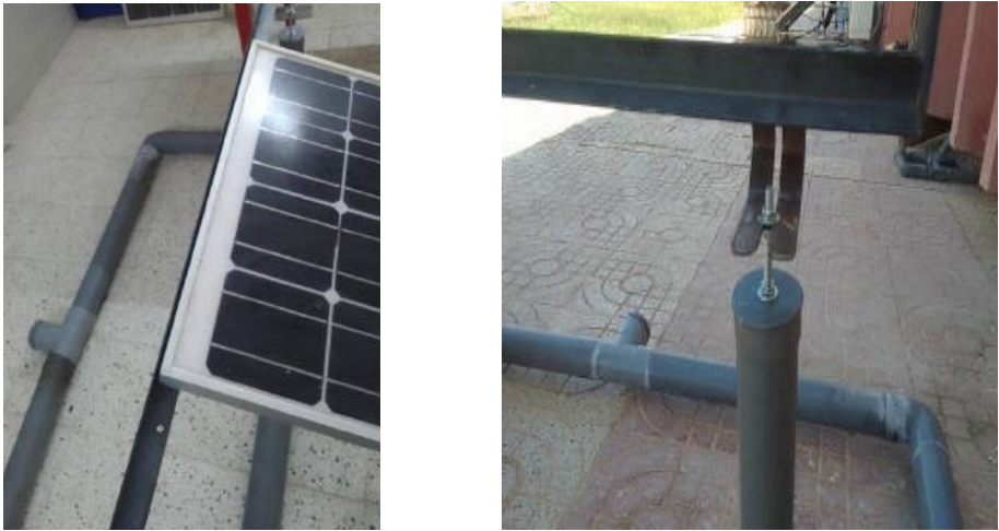
Figure (IV.3). Adjustable Metal Bracket for Solar Panel Mounting on Floating Structure
