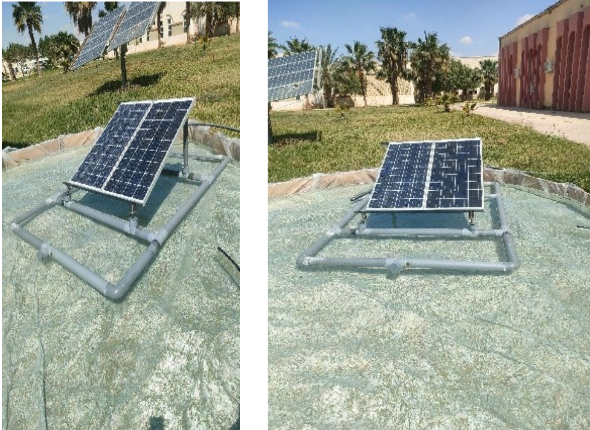
Figure (IV.4). Floating PV Prototype system integrated into an experimental water basin
