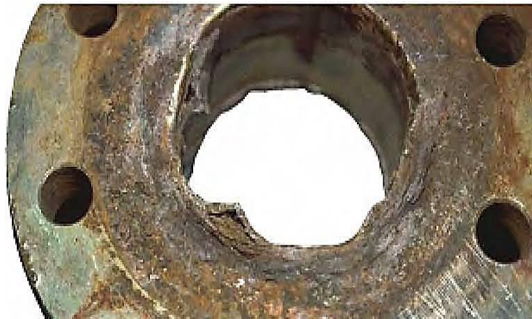
Figure (I.4): La Corrosion Crevasse.
