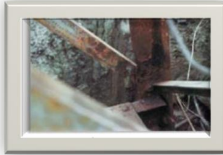
Figure 27 - La corrosion galvanique
