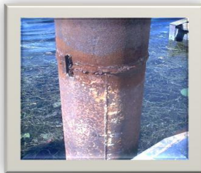
Figure 26 - La corrosion uniforme
