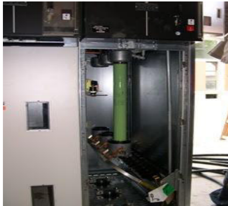
Figure III-18: Porte fusible cellule HTA
