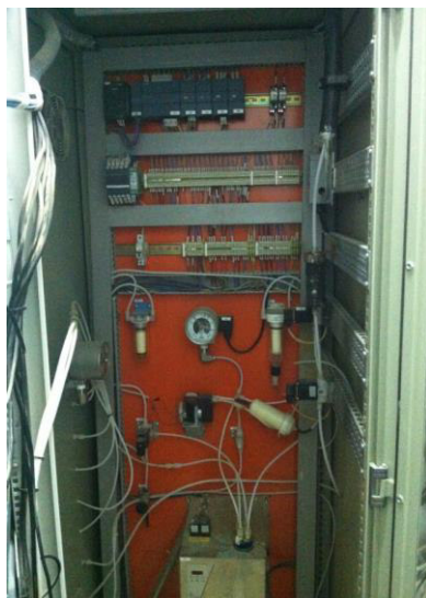
Figure II.8 : Cabinet de commande. [7]
