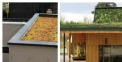
Figure N°51 : Toiture extensive (substrat 6cm) et Toiture intensive (substrat 12 cm)
