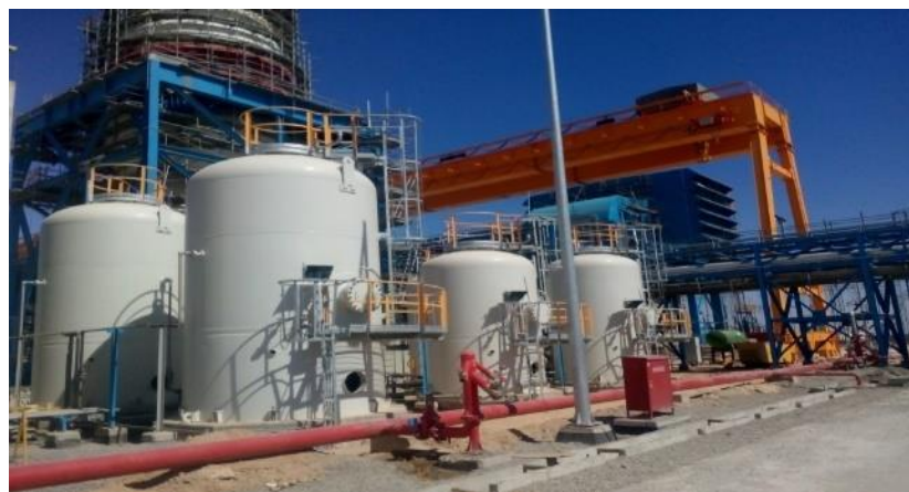
Figure I-4: Station d'air comprimé.
