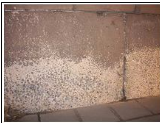
Figure I-12 : Écaillage de surface. [1]
