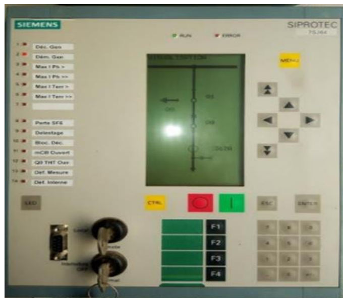
Figure III.24: Relais de protection SIEMENS.
