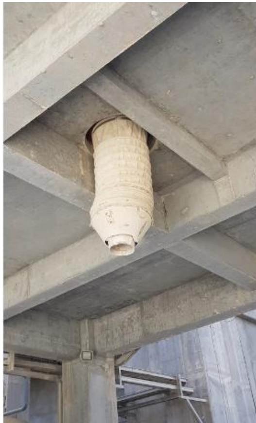
Figure III.2. La bouche vrac
