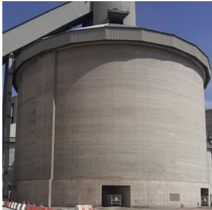
Figure I.15. Silo stockage de clinker
