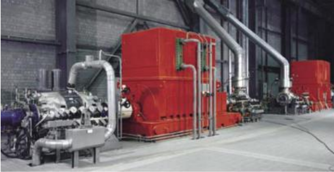
Figure II-1 : Boiler feed pumps in a thermal power plant driven by MEGADRIVE-LCI
