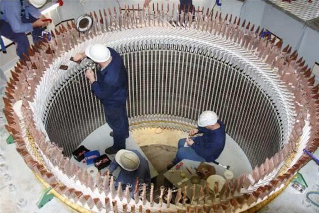
Figure II-22: Typical terminal turns of the stator winding and connections for a hydrogen-cooled bipolar alternator
