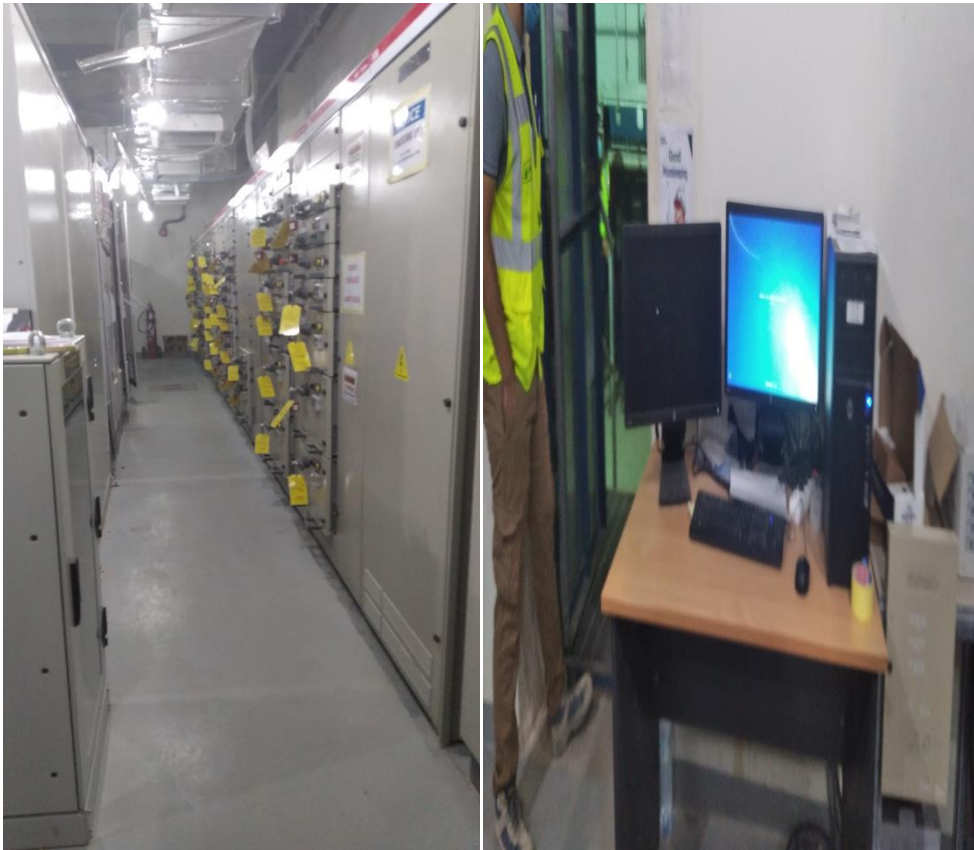
Figure I-3: The electrical room (EROOMS)
