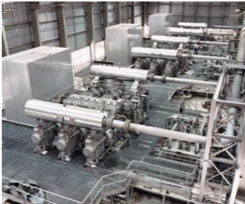
Figure II-2 :Compressor hall with 3 reciprocating compressors equipped with MEGADRIVE-LCI in a natural gas pumping station
