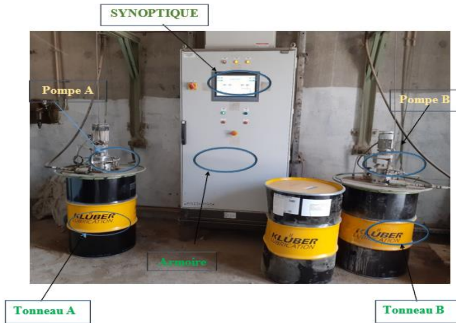
Figure II.1: Unité de lubrification
