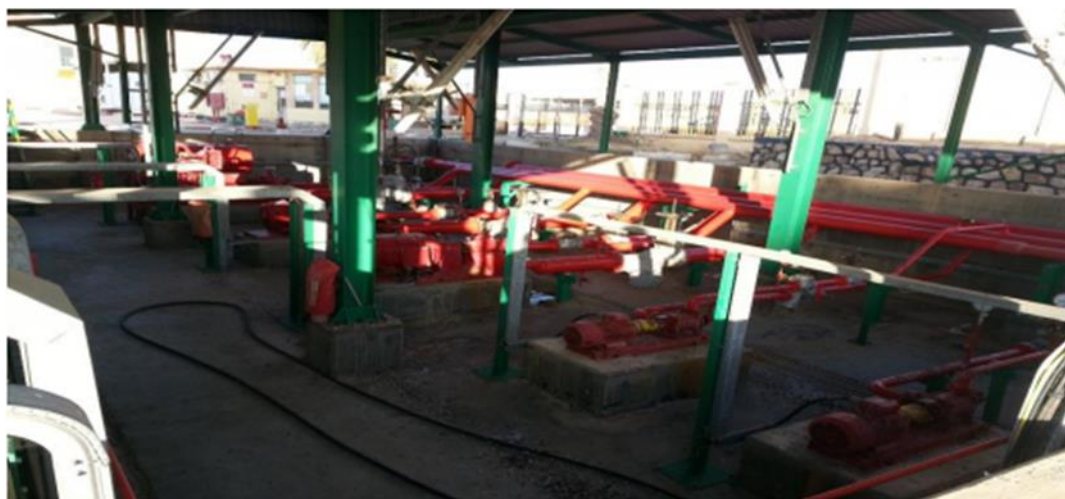
Figure I.25. Centrale anti- incendie.
