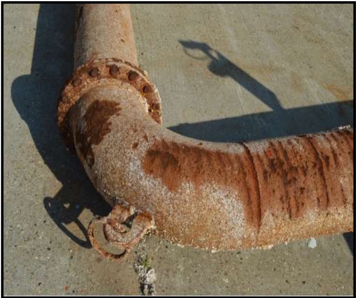
Figure I- 5 : Image de corrosion uniforme [13].
