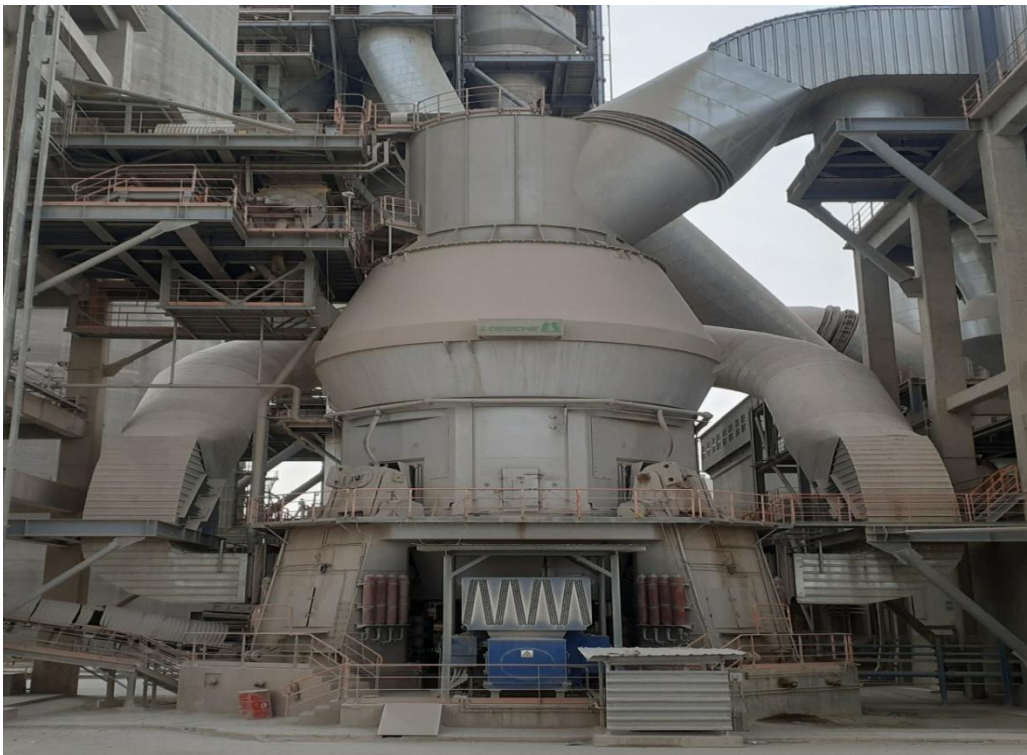
Figure I.10: Broyeur cru vertical
