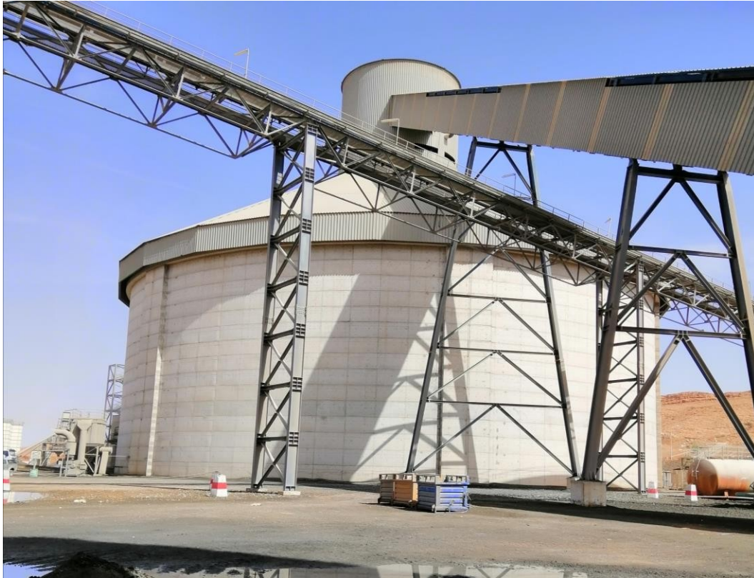
Figure I.13: Silos stockage de clinker.
