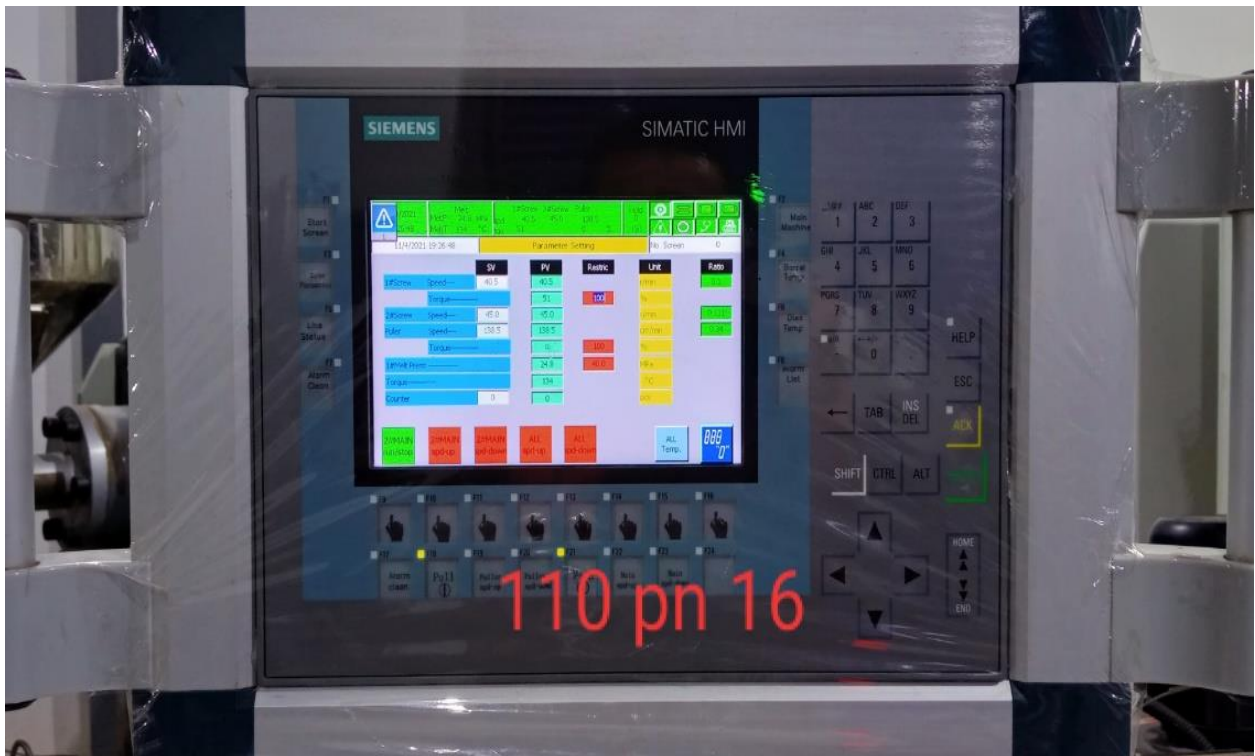
Figure 3.11. HMI KTP700 Confort [14]
