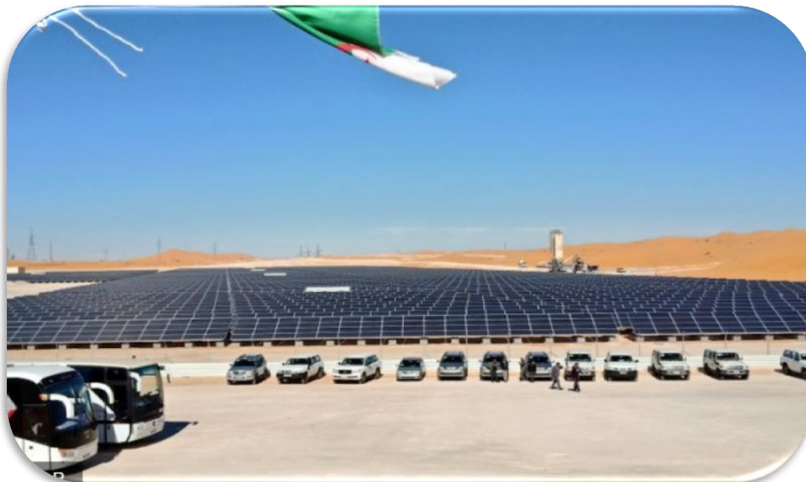
Figure I.15: La centrale PHOTOVOLTAÏQUE
