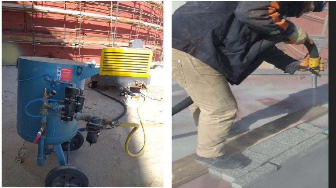
(a) Sandblasting machine
