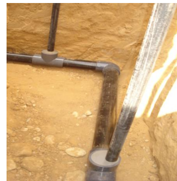
Figure 5. Location of RTD temperature sensors in the buried pipe.
