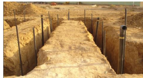
Figure 4. General view of the EAHE.
