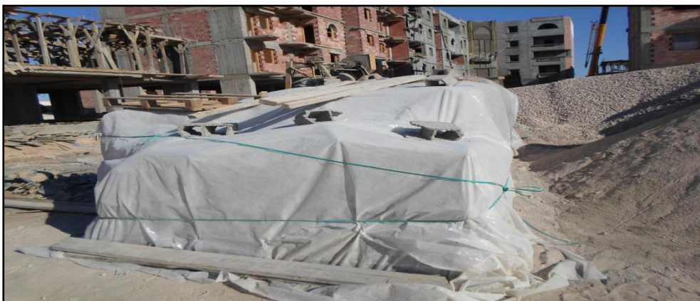
Figure 11: stockage du ciment
